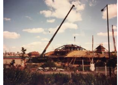
"The Boathouse" under construction in late 1989 - to house the new marina's offices, coffee shop and chandlery, which opened on April 11th 1990.
